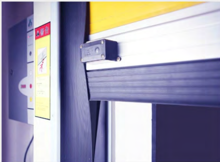
New aluminum alloy integral bottom beam installed with safety rubber protection device.
