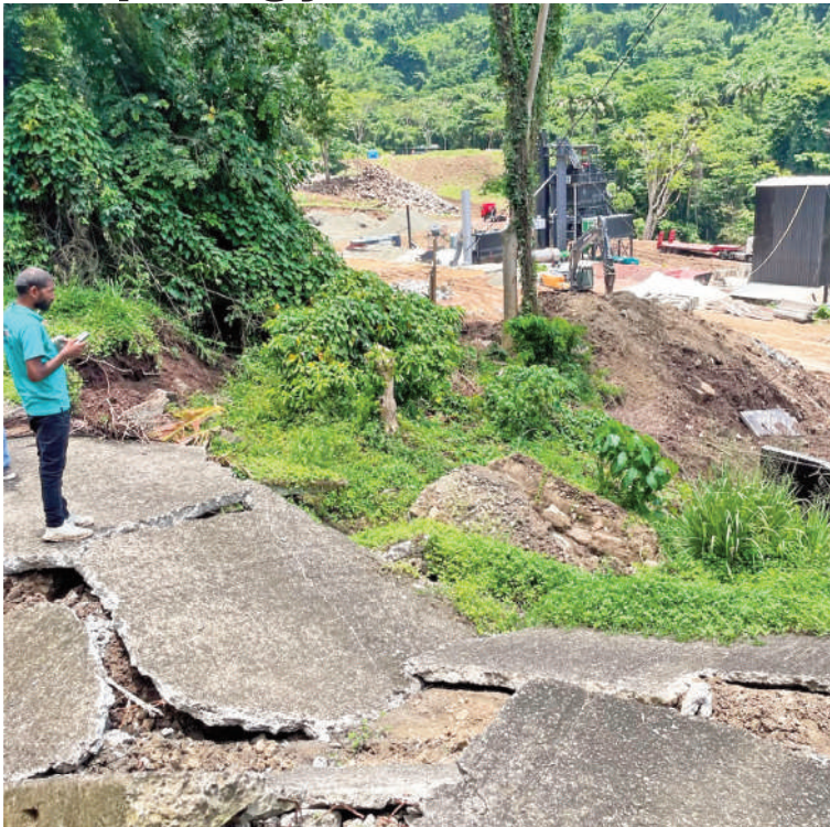
A worker surveys the broken Mt. Dor Farm Road, with the Rayneau plant almost directly in line with the road below. Once motorable, the road has now failed at three points along the stretch bordering Rayneau's Woodford operations, disrupting access to homes and agricultural lands
