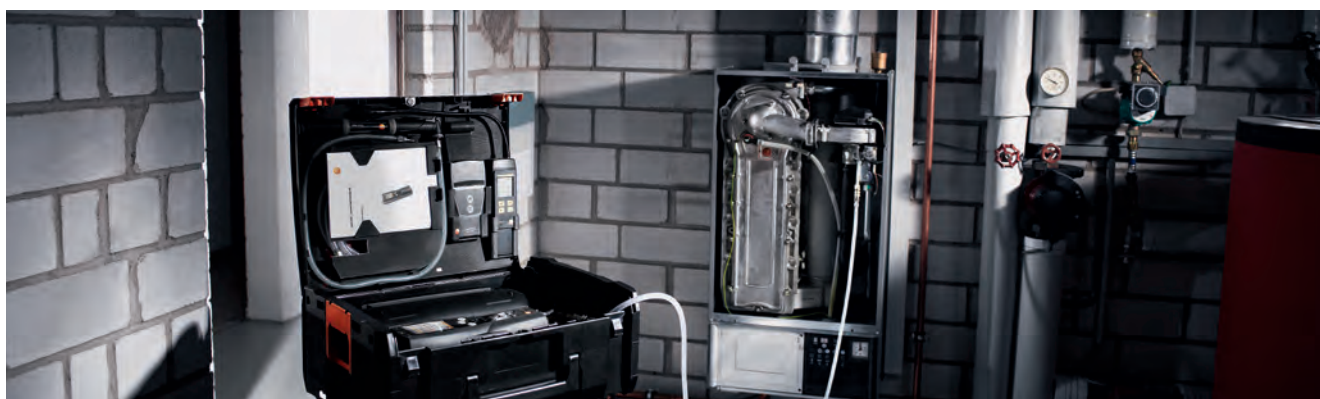
Automatic servicability test with gas-feed appliance with connection to the gas boiler
