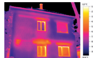
Thermal image with ScaleAssist
