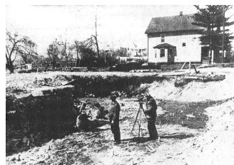
CROSSING STRATFORD AVE. the roadbed plows on toward a row of marked houses.
