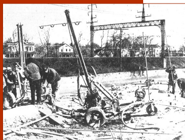
THE ROCK never has a chance against this team of blasters in Church St. The hole drillers...work a few yards ahead of the crew that charges the hold. After a steel cover is placed over the area, the blast is set off.
