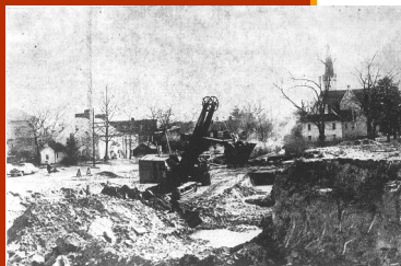
Thuway Construction Makes Big Dent in Church Street. POWER SHOVELS working in Church St. this week produced this gaping hole, as they cleaned up behind the blasting crews.
