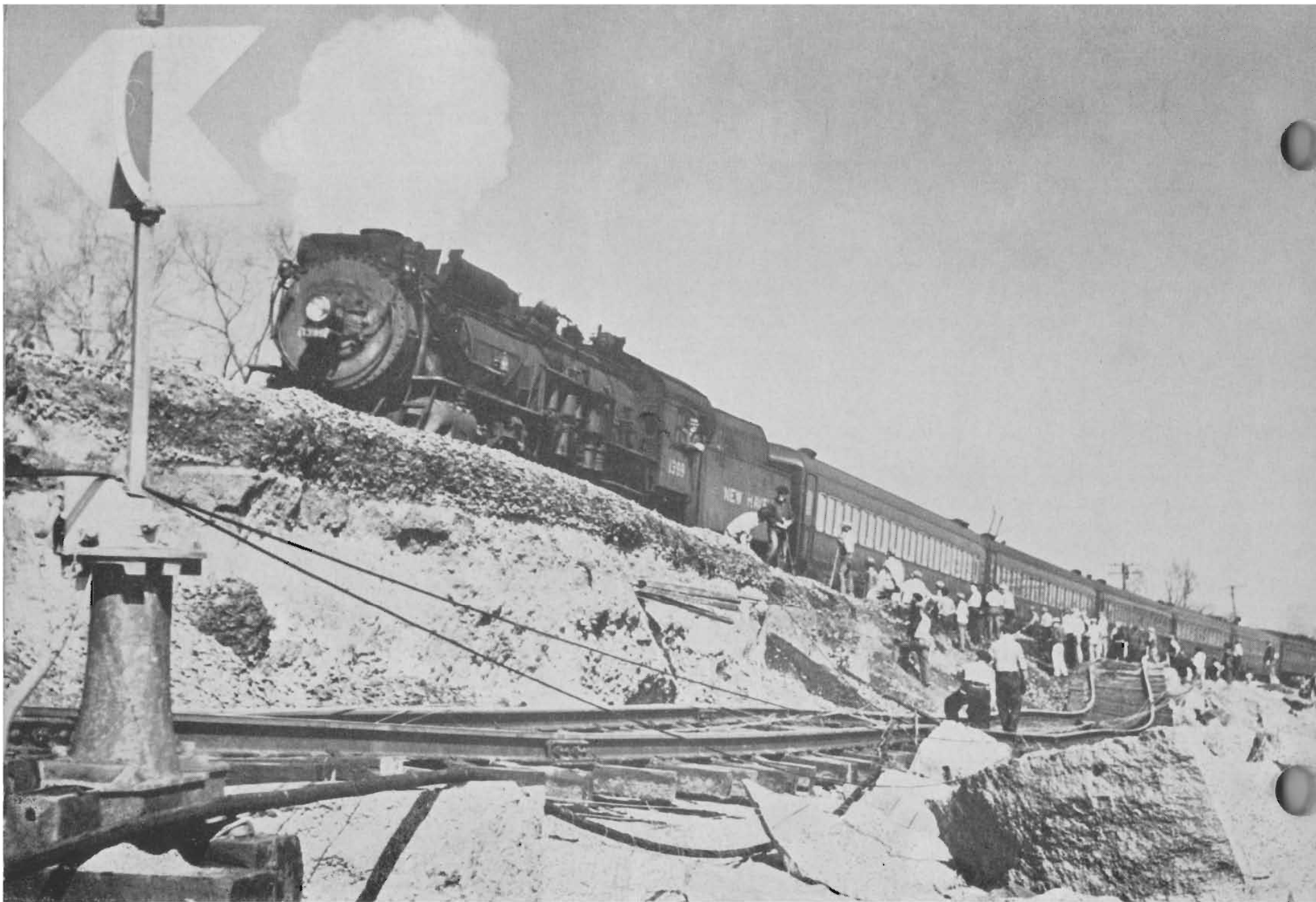
Restored rails were tested by work trains . . . followed first by freight trains carrying emergency supplies and vital necessities . . . then by passenger trains in partial single track service along the Shore Line.
