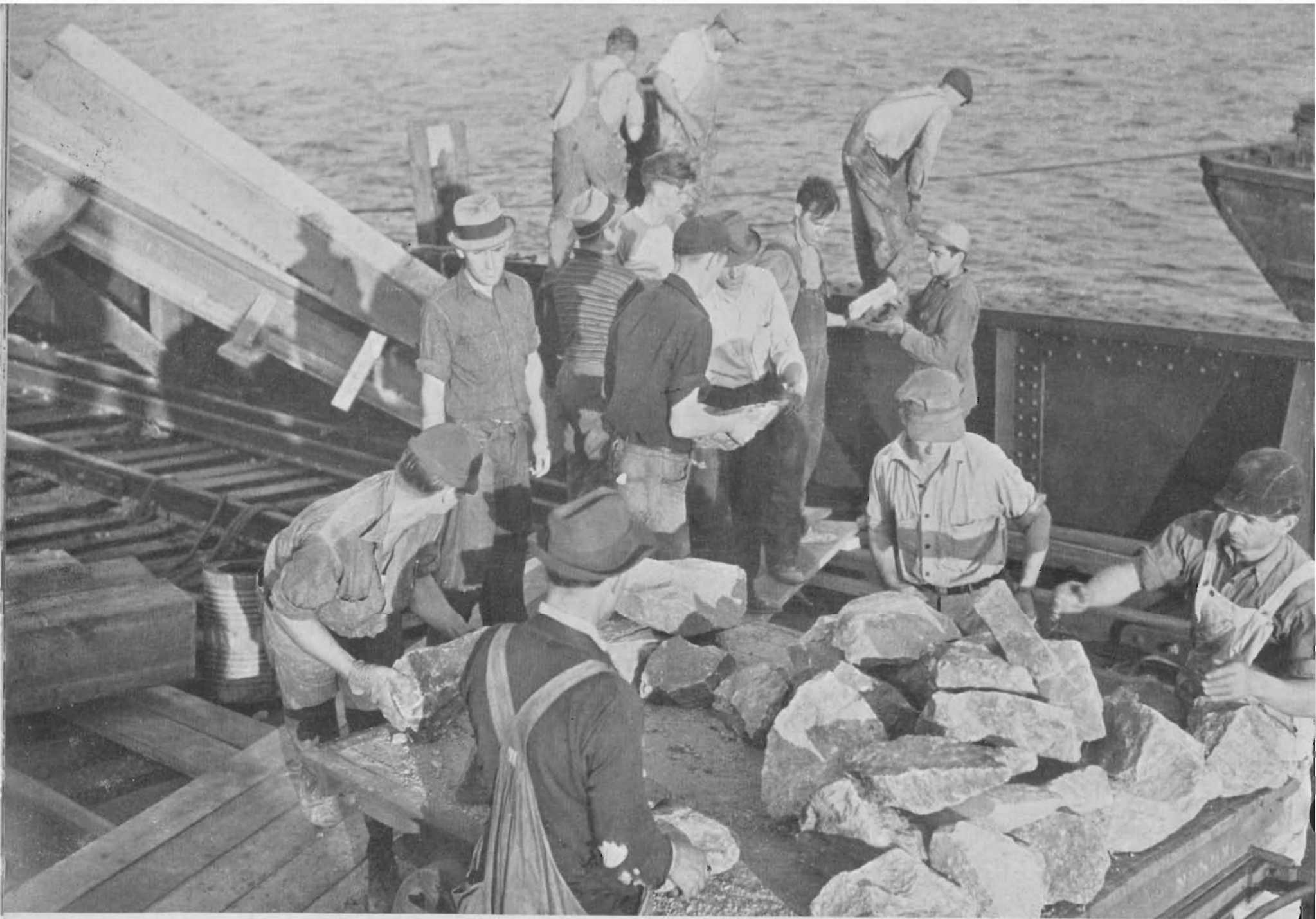
TONS OF RIP-RAP are required to hold cribbing support for bridge while piles are being driven.
