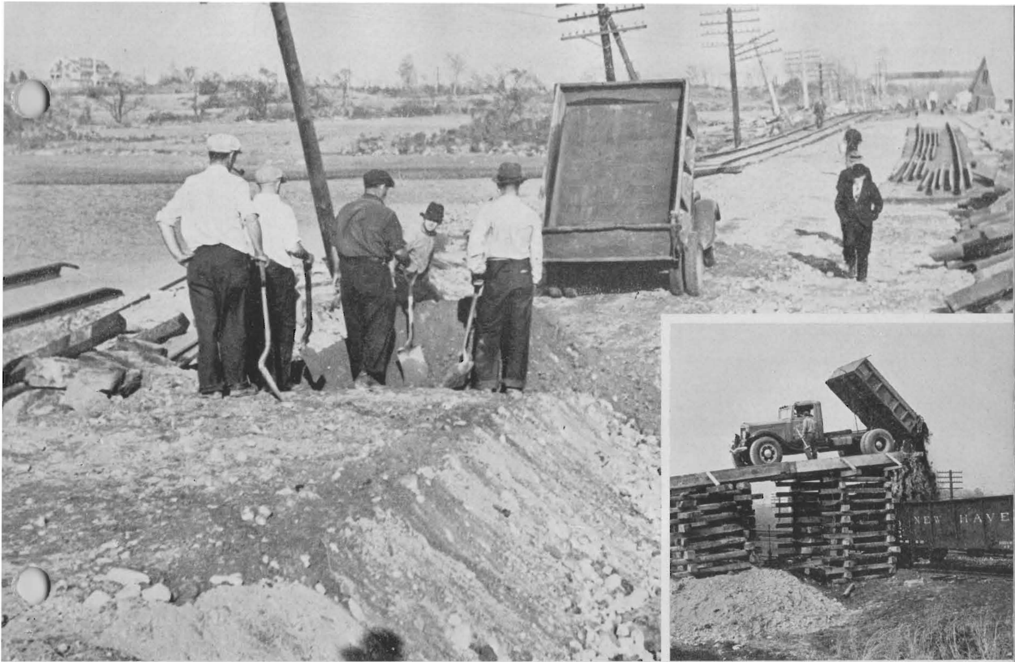
In several areas complete road beds must be replaced and miles of track re-laid.
