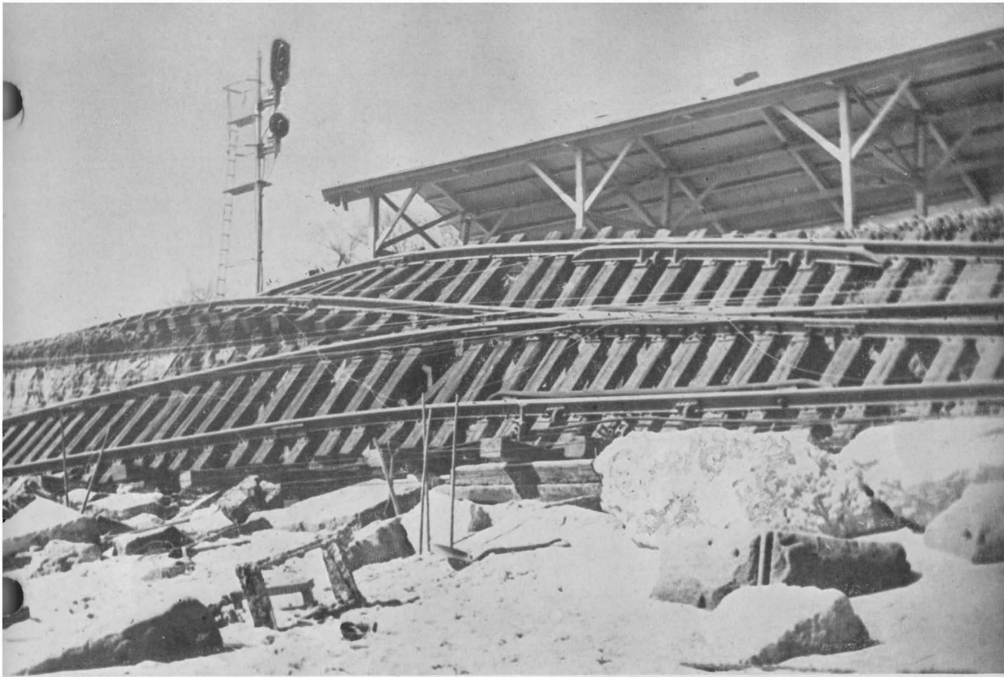
NIANTIC . . . Thirty foot embankment completely washed out . . . all telegraph poles and wires down.
