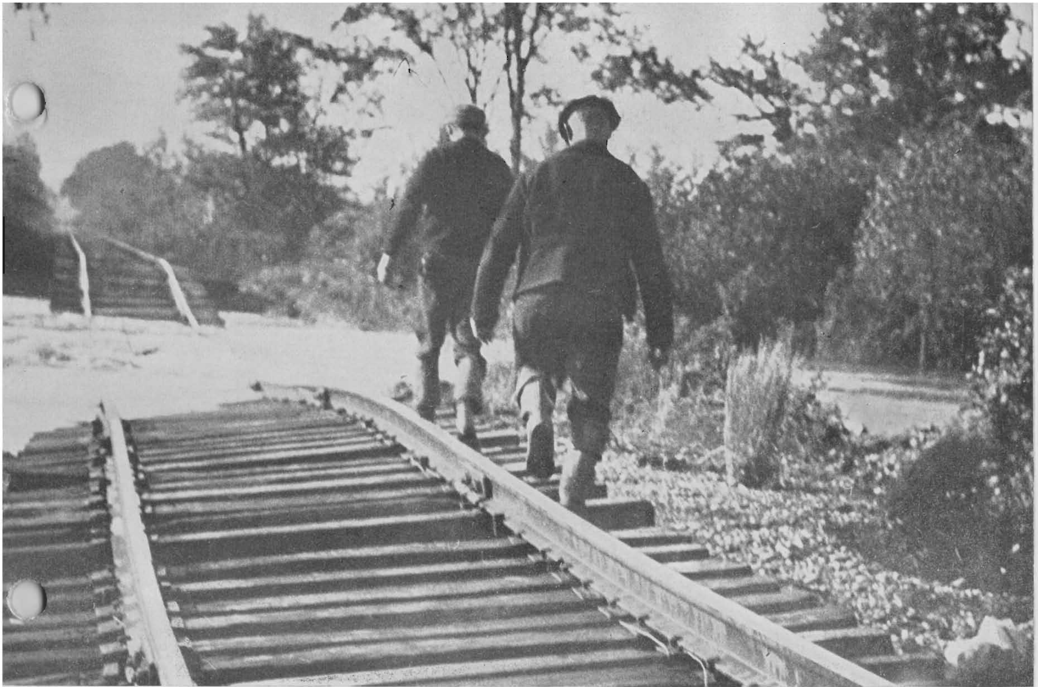
GREAT BARRINGTON . . . Washouts and twisted rails at the junction of the flooded Housatonic and Green rivers.
