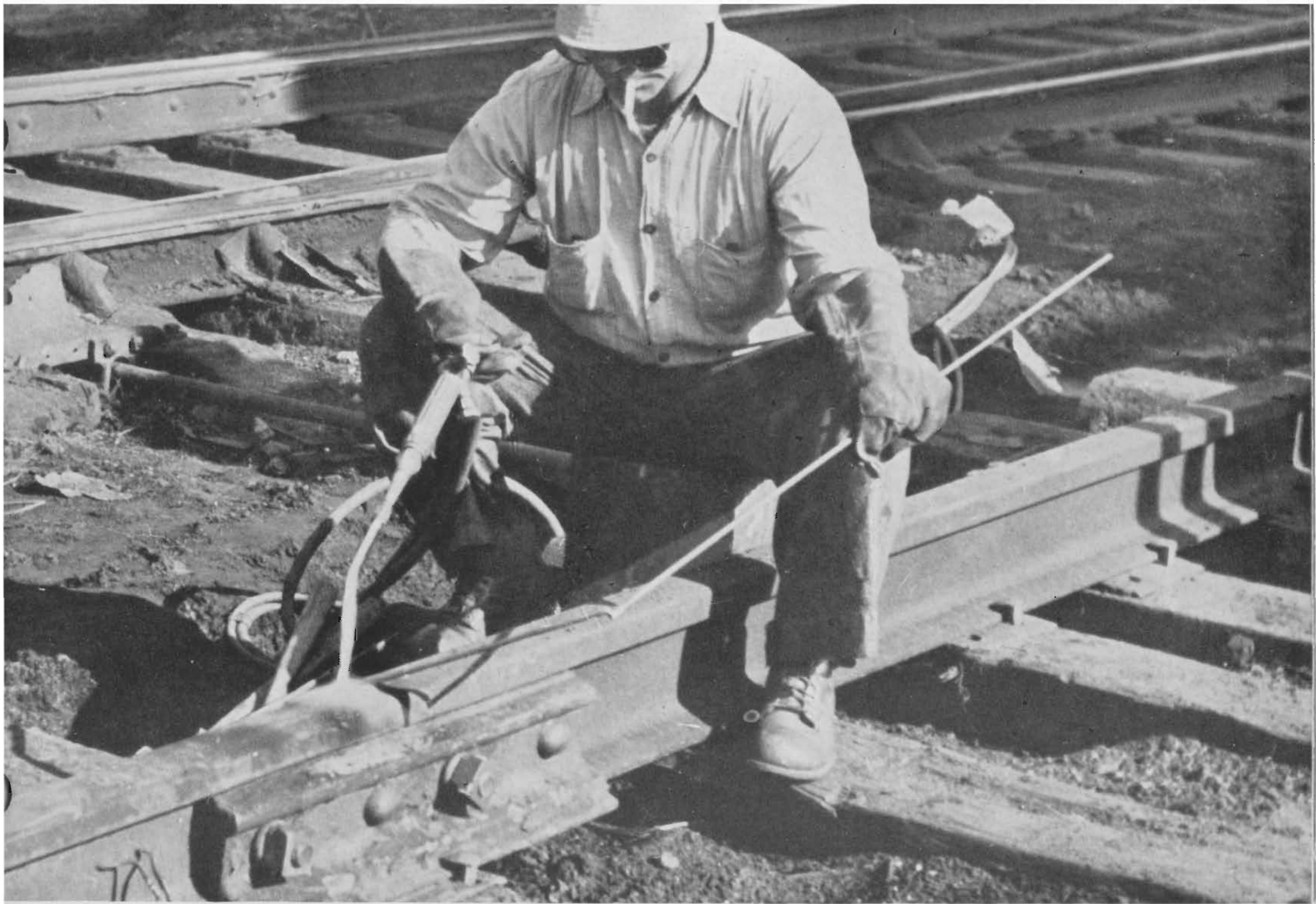
WELDERS and grinders restore the reset Shore Line rails to their original smoothness and finish.
