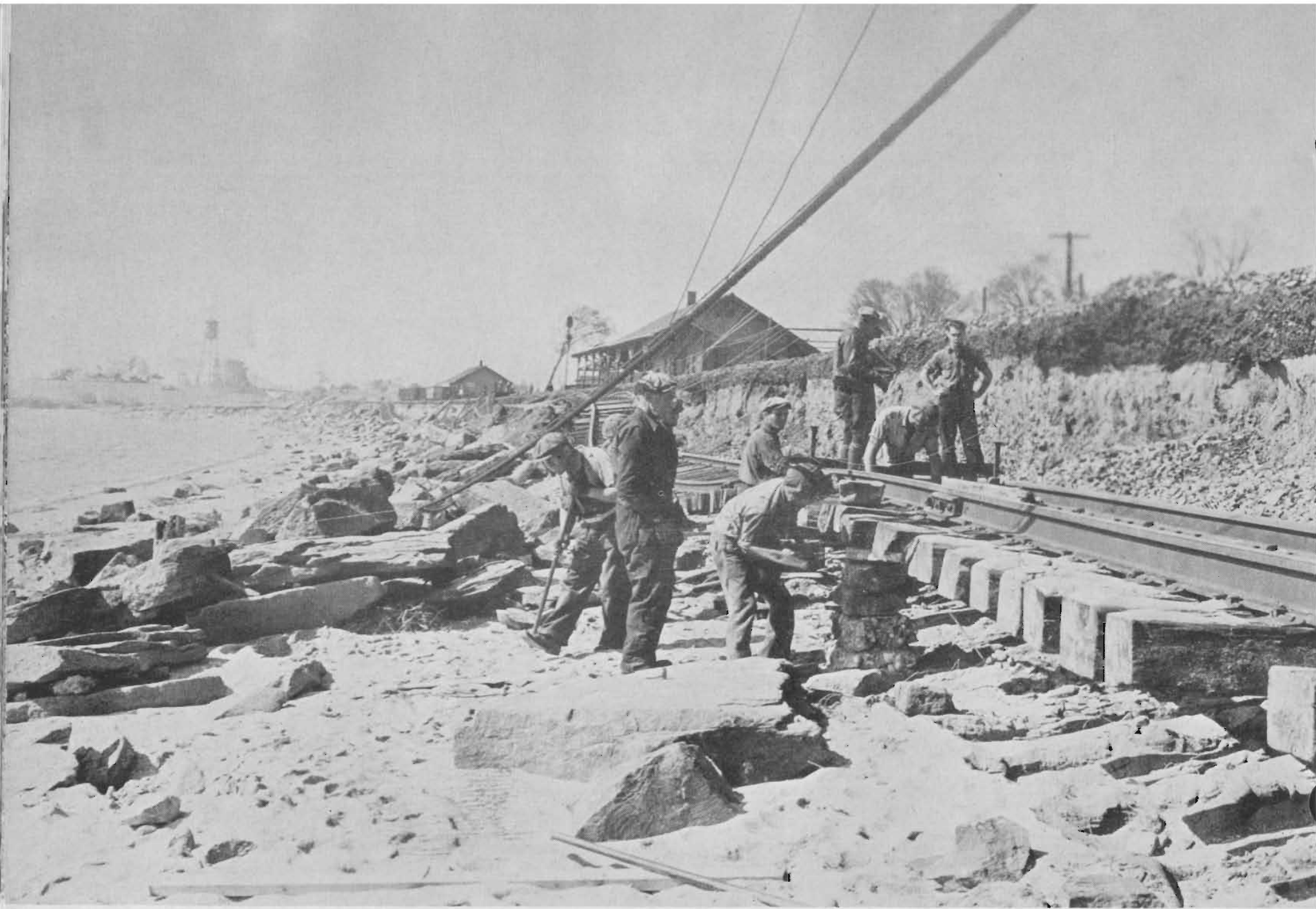
EASTBOUND TRACK must still be built up some 6 feet to meet the level of the westbound track.
