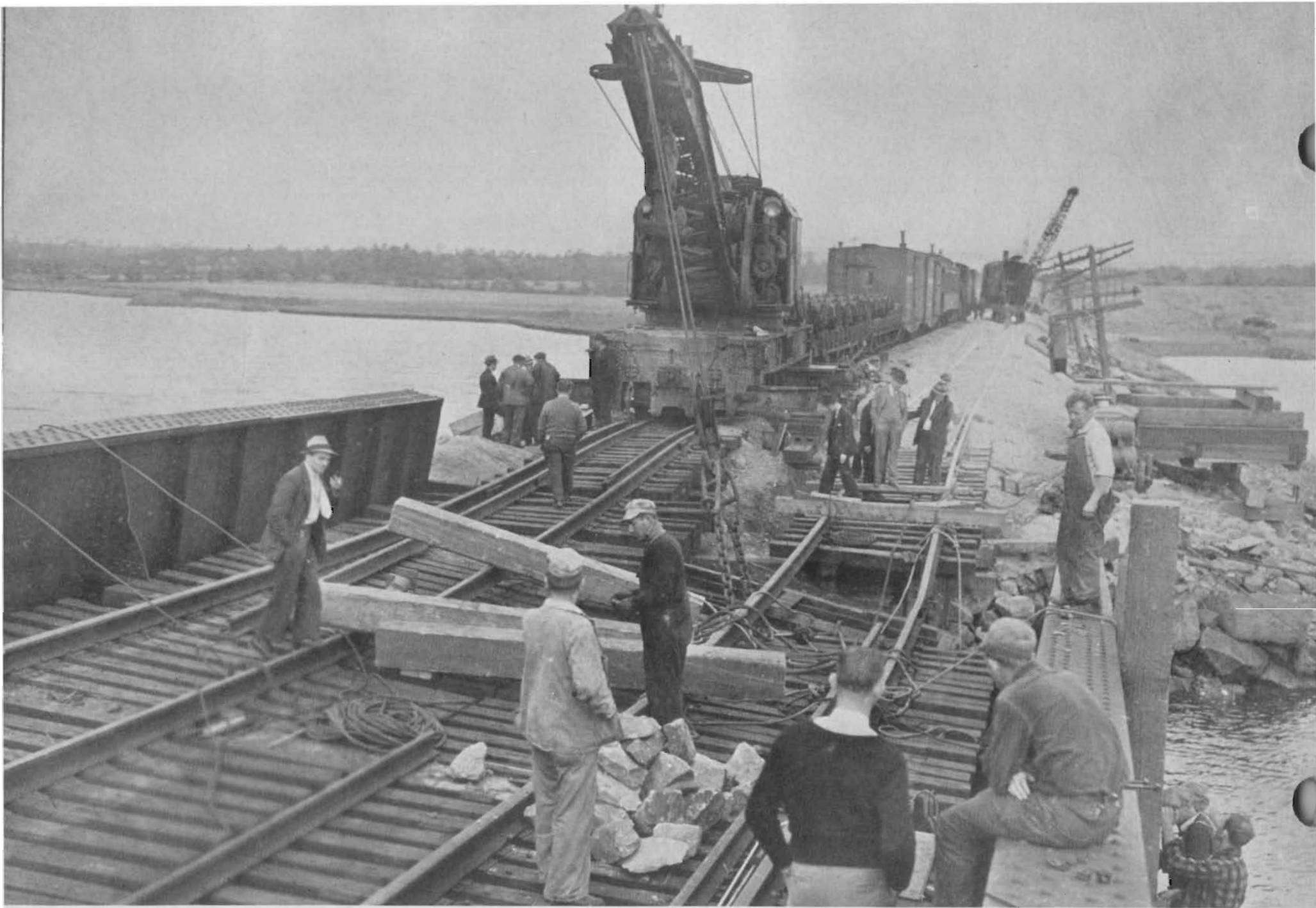
ONE OF THE 31 washed-out bridges is temporarily held in position by a giant crane while engineers figure out ways
