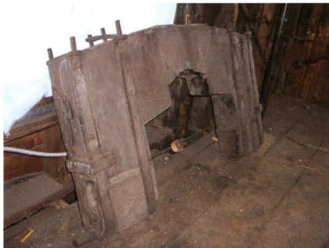
The ancient church bell yoke which now sits in the upper reaches of the steeple. How much ringing did these timbers absorb in the last 150 years?
