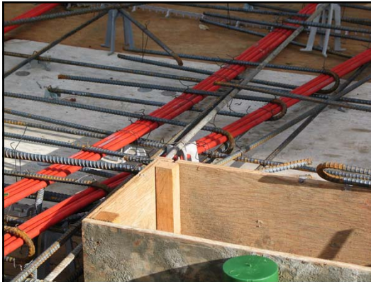
In this detail hairpins restrain the tendon from causing blowout
