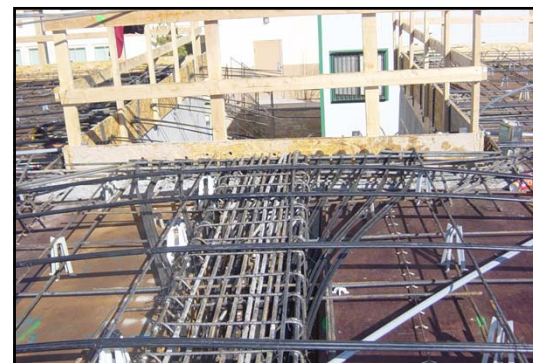
Beam tendon diverted into the slab without adequate restraint
