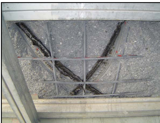
Looped tendon not adequately secured in plane of the slab slipped out of position at bottom of slab upon removal of forms.
