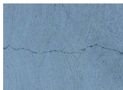
Long deep restrain cracks
