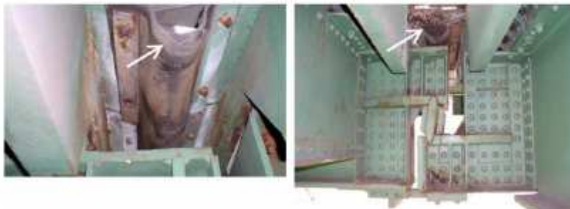
Clogged elastomeric through on Gerber joint in steel girder.
