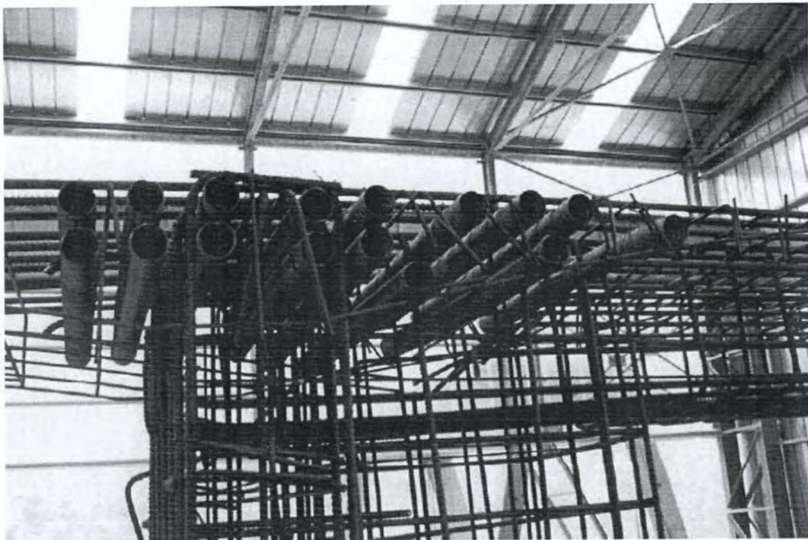
As regards formwork, the pictures show details about the front, the reinforcement cage made of welded reinforcement and the tubes to insert tendons.
