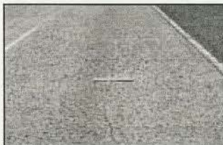
Figure 94 Distress Type CRCP 2—Low Severity Longitudinal Cracking
