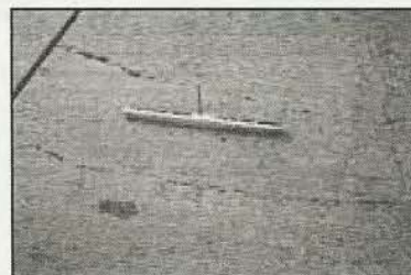
FIGURE 124 Distress Type CRCP 12—Low Severity Punchout
