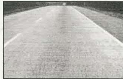
FIGURE 101 Distress Type CRCP 4a—Map Cracking Attributable to Alkali-Silica Reactivity
