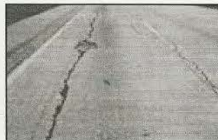
FIGURE 95 Distress Type CRCP 2—High Severity Longitudinal Cracking
