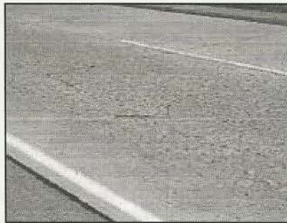
FIGURE 56 Distress Type JCP 3—Moderate Severity Longitudinal Cracking
