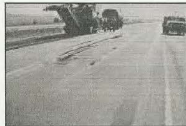
FIGURE 33 Distress Type ACP 9—Standing Water in Ruts
