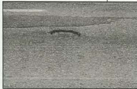
FIGURE 28 Distress Type ACP 8—Moderate Severity Pothole
