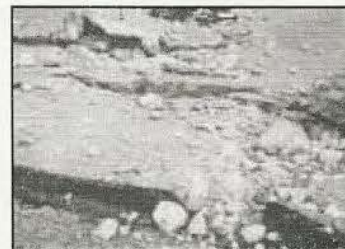
FIGURE 108 Distress Type CRCP 7—Close-up View of a Blowup
