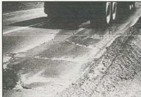
FIGURE 89 Distress Type JCP 16—Water Bleeding and Pumping
