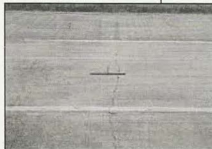
FIGURE 99 Distress Type CRCP 3—Moderate Severity Transverse Cracking
