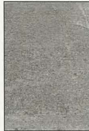
FIGURE 102 Distress Type CRCP 4b—Scaling
