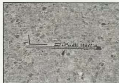
FIGURE 74 Distress Type JCP 10—A Popout
