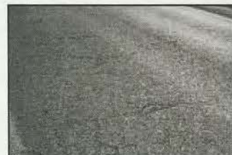
FIGURE 10 Distress Type ACP 2—High Severity Block Cracking
