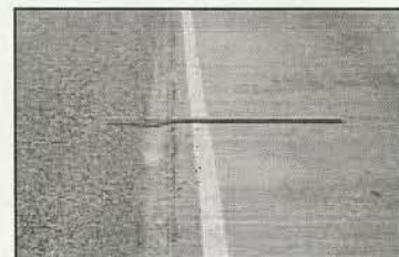
FIGURE 115 Distress Type CRCP 9—Lane-to-Shoulder Dropoff
