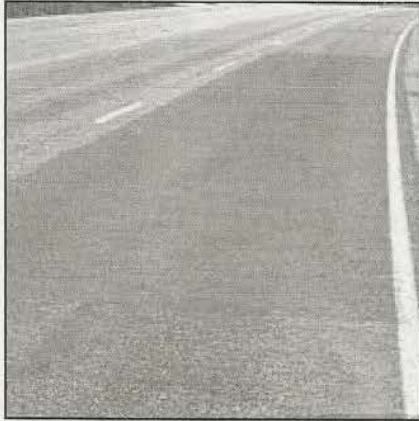
FIGURE 23 Distress Type ACP 7—Low Severity Patch
