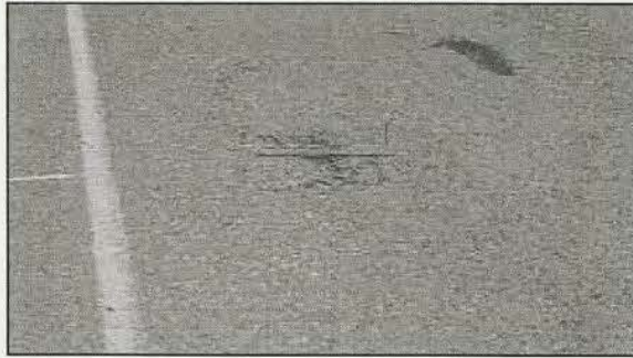
FIGURE 27 Distress Type ACP 8—Low Severity Pothole
