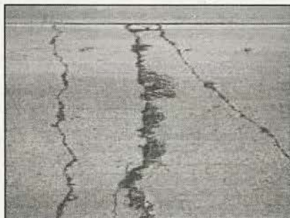
FIGURE 100 Distress Type CRCP 3—High Severity Transverse Cracking
