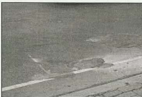
FIGURE 25 Distress Type ACP 7—High Severity Patch
