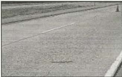
FIGURE 55 Distress Type JCP 3—Low Severity Longitudinal Cracking
