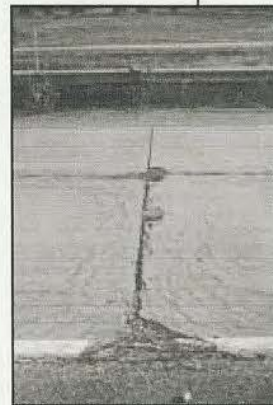
FIGURE 53 Distress Type JCP 2—High Severity "D" Cracking with Loose and Missing Material
