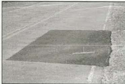
FIGURE 24 Distress Type ACP 7—Moderate Severity Patch
