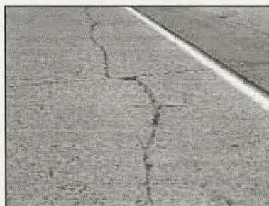
FIGURE 57 Distress Type JCP 3—High Severity Longitudinal Cracking
