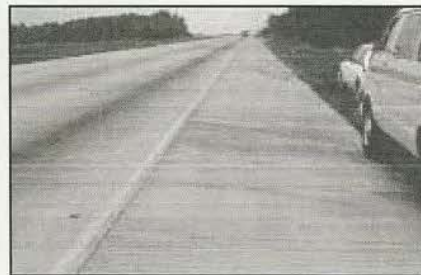
FIGURE 131 Distress Type CRCP 14—Water Bleeding and Pumping
