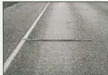
FIGURE 32 Distress Type ACP 9—Rutting
