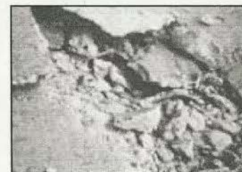
FIGURE 109 Distress Type CRCP 7—Exposed Steel in a Blowup
