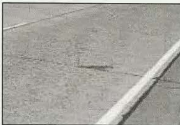
FIGURE 67 Distress Type JCP 7—Moderate Severity Spalling of Transverse Joint, Far View
