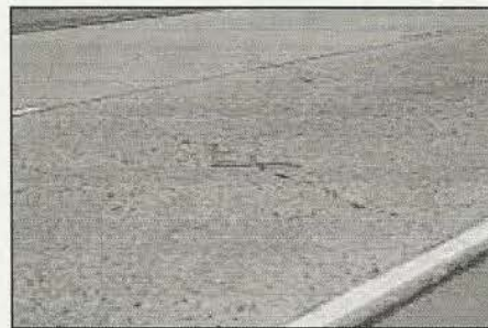
FIGURE 60 Distress Type JCP 4—High Severity Transverse Cracking
