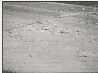
FIGURE 107 Distress Type CRCP 7—A Blowup
